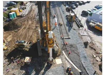
Crews drilling to construct the east foundation for the future light rail bridge over Foothill Blvd./Grand Ave.
