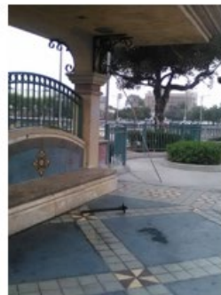
Transit Center Theft of electric wires
