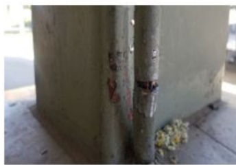
Ganesha Park Band Shell – Conduit damage from wire theft
